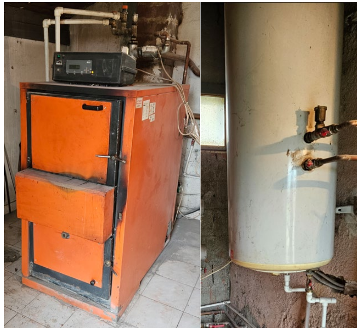
Figure 2. School from Romania – heating source
